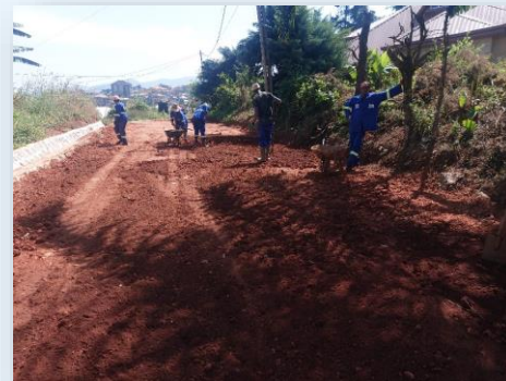
Backfill from borrow pit being leveled on the road using the traditional method (PK 0+385 that's besides court of first instance) (ILO).
