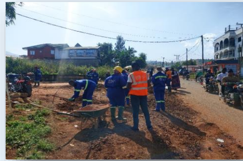
Cuts being performed on the road using the traditional method (PK 0+000 that's opposite transport office) (ILO).
