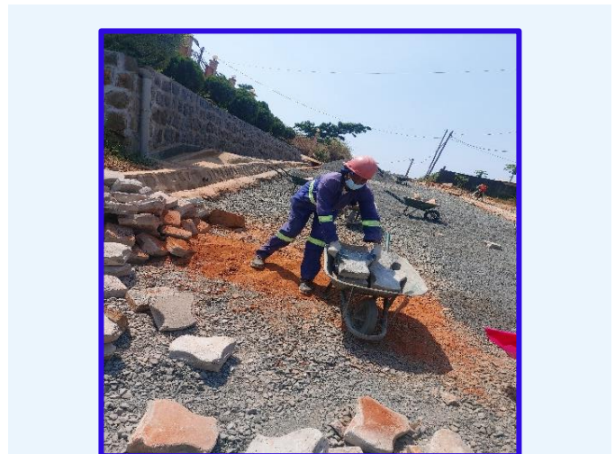
Madam Nfor Jackline serious at her wok carrying pavement blocks for laying (ILO).
