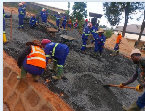
Backfill with crushed gravel from quarry trainees taking levels being leveled on the road using the traditional method (PK 0+050) (ILO).
